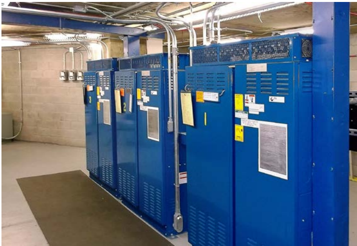
Photo #42 Elevator controllers – typical for six elevators – three per tower. An elevator modernization was performed in 2008 including upgrade to A.C. lift motors controlled by VFDs. The equipment appeared to in good overall condition.
