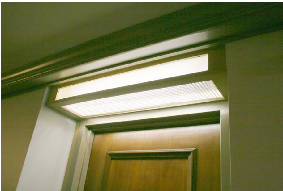
PHOTO #22 As part of the corridor restoration project, “top hat” lighting fixtures will be installed above all unit doors. This will be a welcome improvement to the overall lighting situation of the corridors.
