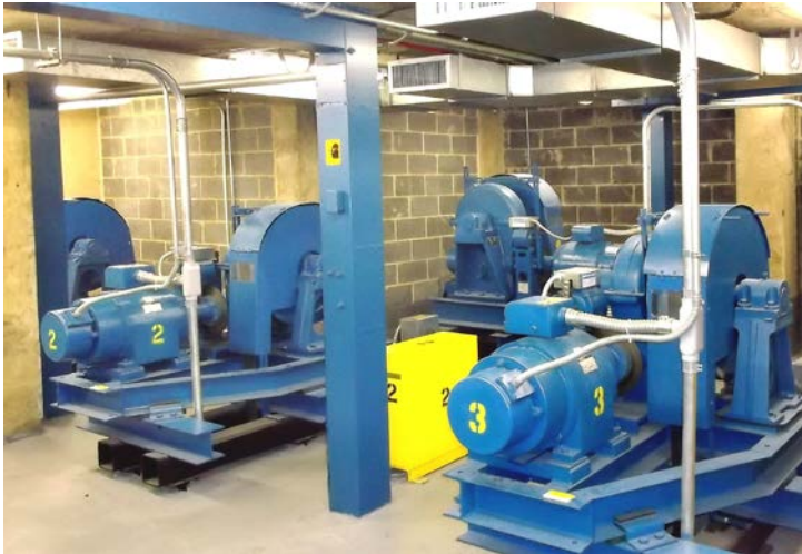
Photo #41 Elevator lift machinery – typical for six elevators – three per tower. An elevator modernization was performed in 2008 that included lift machinery replacement. The equipment appeared to in good overall condition.
