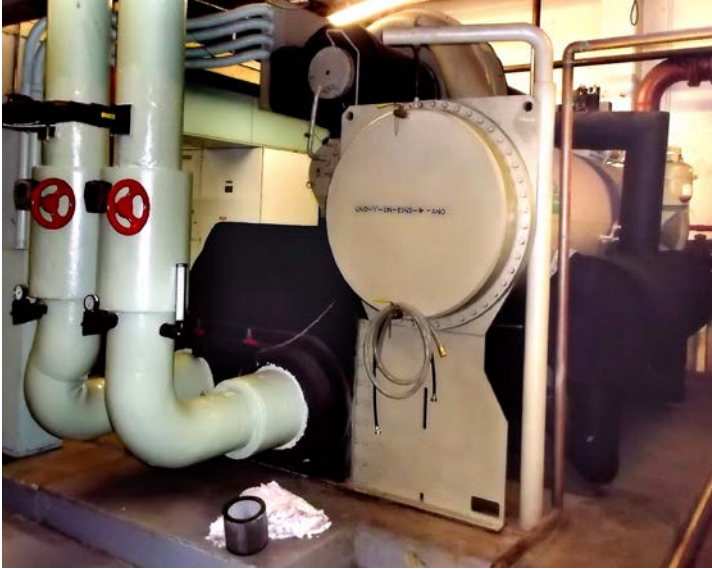
Photo #40 One of two main water chillers. They were replaced in 1996 and appear to be in good overall condition.
