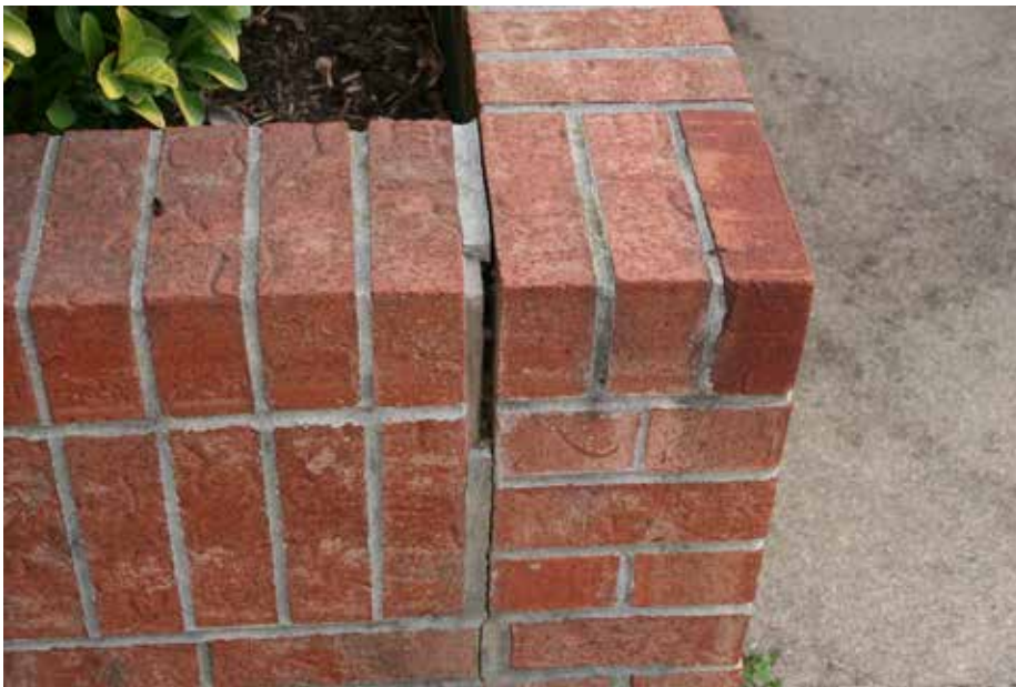
PHOTO #23 Additional tuckpointing and masonry repairs/waterproofing of planters will be necessary on an on-going basis, and we have programmed the component accordingly.
