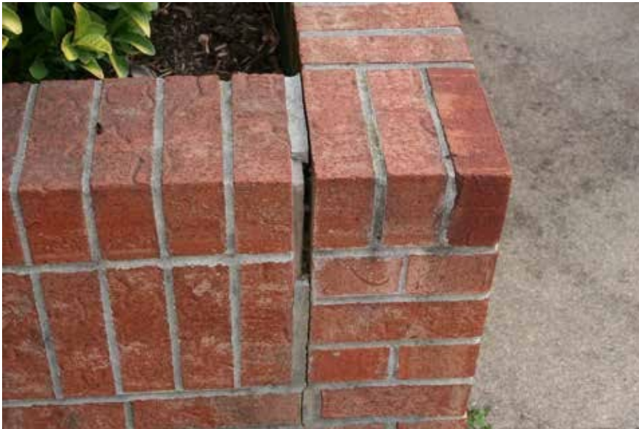
PHOTO #23 Additional tuckpointing and masonry repairs/waterproofing of planters will be necessary on an on-going basis, and we have programmed the component accordingly.
