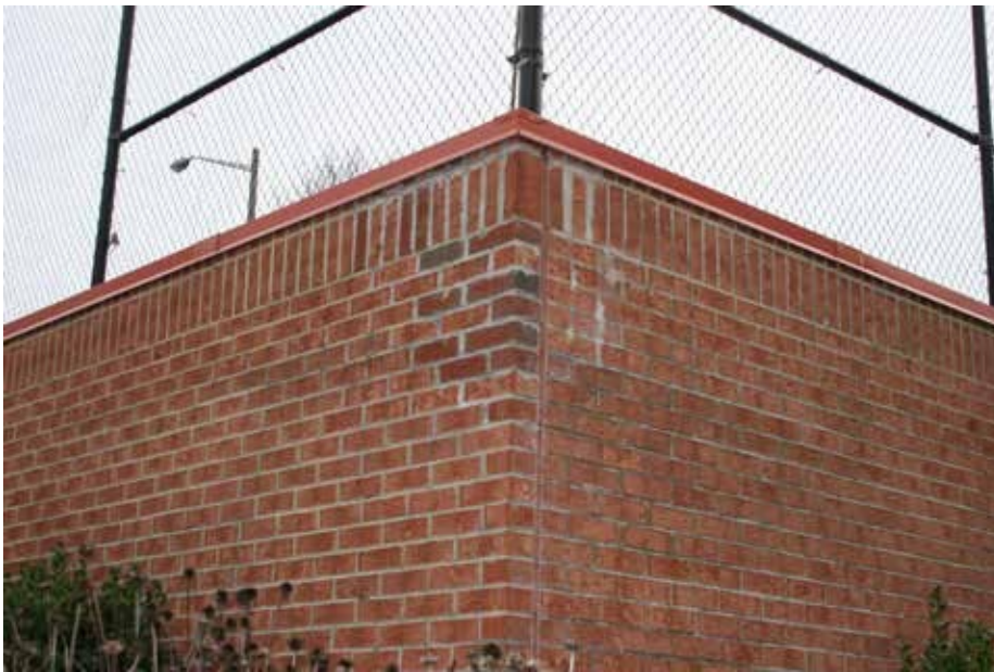
PHOTO #22 The 2007 recommended engineered repairs to the masonry retaining wall appear to have been successful.
