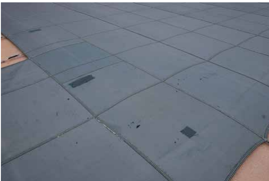
PHOTO #24 The pool cover is aging and tired. We have scheduled replacement in 2013.
